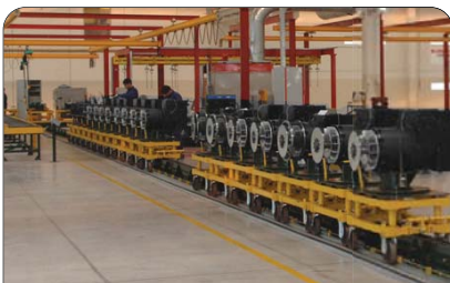
Routine testing at full load and overspeed of the totality of the alternators
